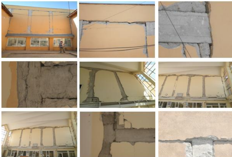
Figure 4. Damage to column-beam joints and walls in the second block [9]
